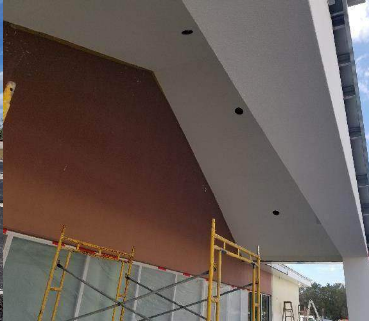
Portico Ceiling Complete
